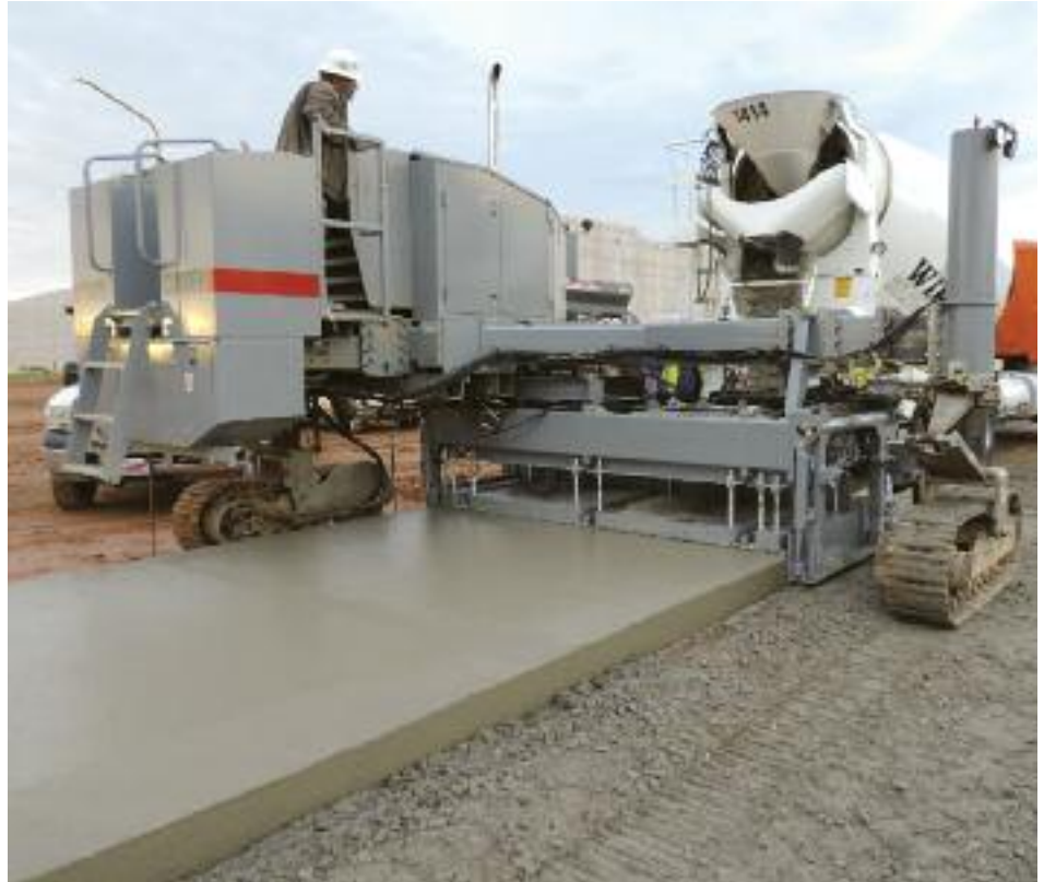
Center pour paving 10' (3m) wide. Concrete is dumped directly into a hopper at the front of the paving mold.
