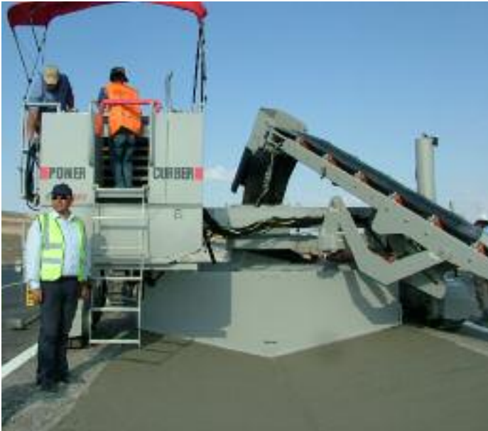
Ditch Liner in Turkey, 12.5' (3.8m) wide and 2' (.6m) deep, adjacent to pavement on both sides. (shown with custom belt conveyor)
