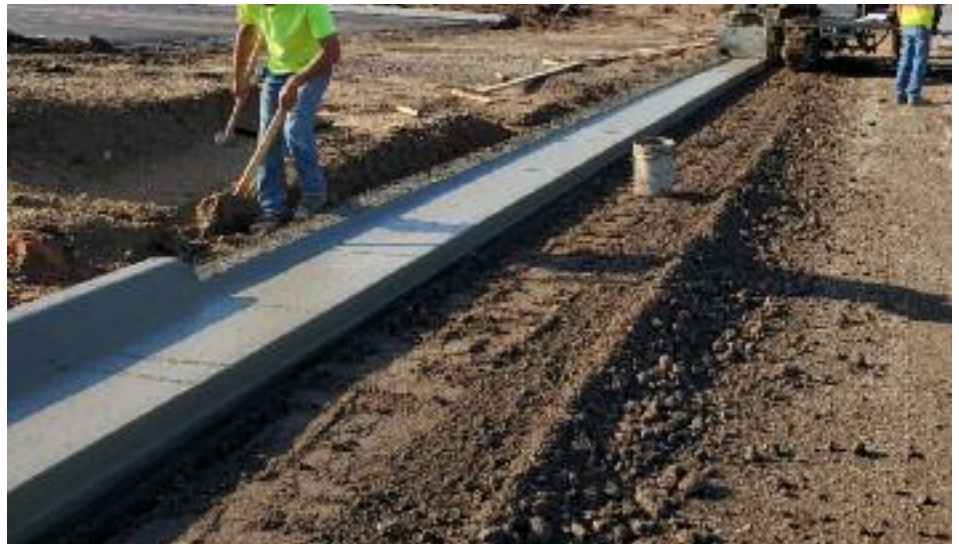
Driveway knives reduce wasted material and labor. Some hand finishing is required.
