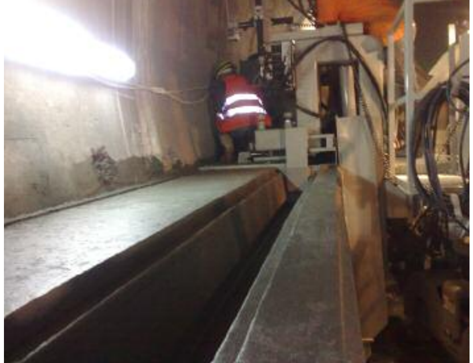
Platform & wall structure poured along a tunnel wall in Turkey – mold is adjustable in height and width to accommodate varying tunnel diameter.
