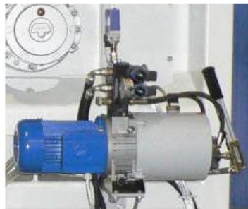
Emergency hydraulic door opening.
