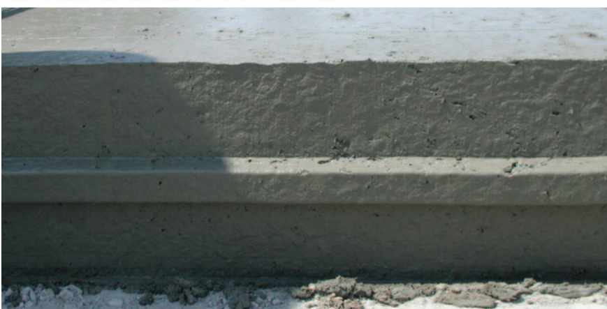
Edge of pavement with optional key-way inserter (top), and optional male key-way block-out (bottom).
